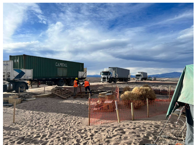
Figures 3 & 4: Demonstration Plant
