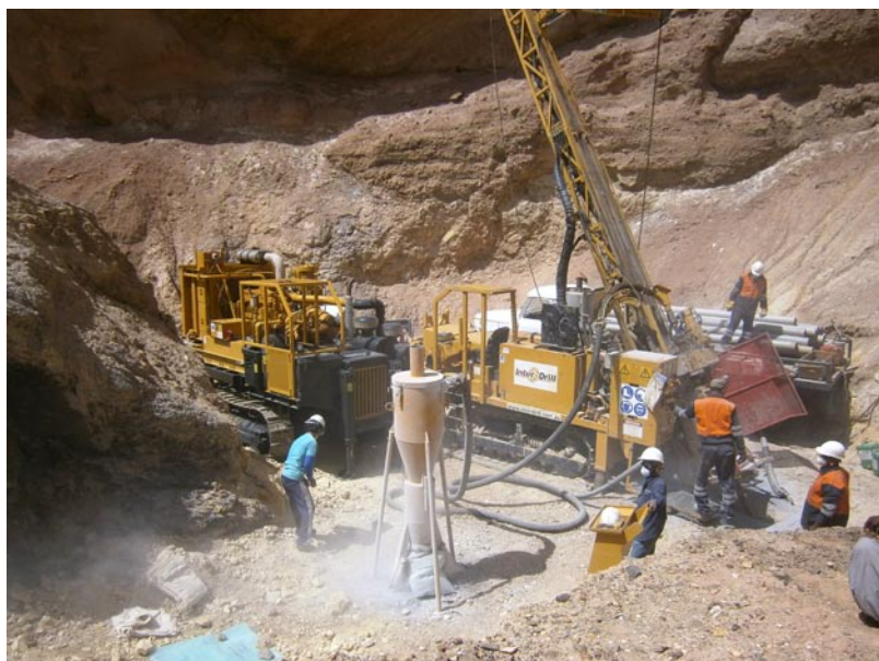
Figure 4: Drill Site LRMRC-003 Crawler-mounted compressor on left, multi-purpose drill centre and cyclone sample collector front-centre.
